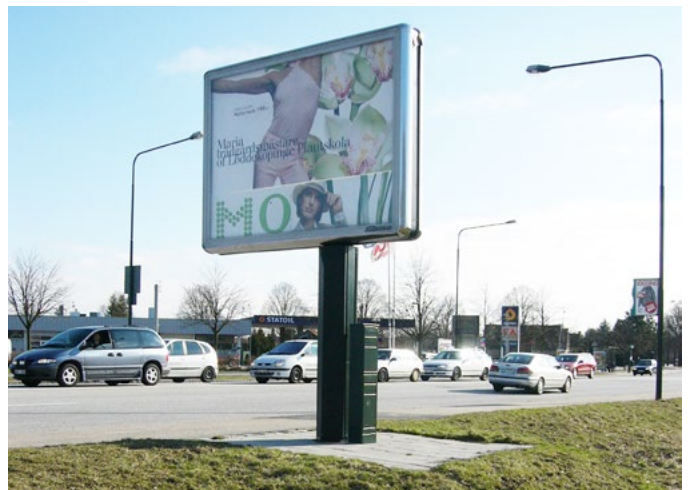
Cable distribution board for illuminated advertising signs.
