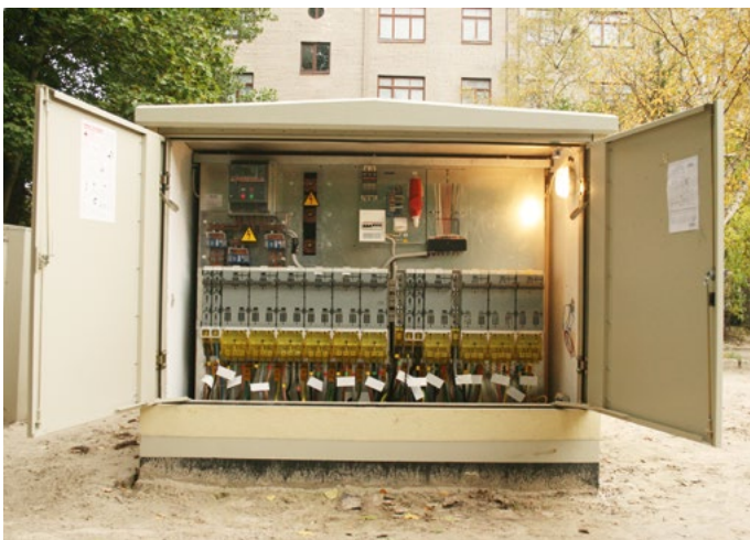
Kabeldon switching devices in a CSS, Latvia.
