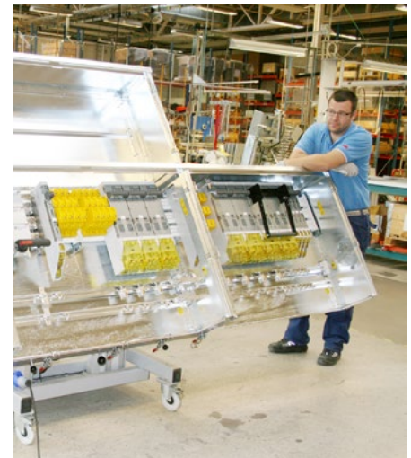
Assembly of distribution boards according to customer specific requirements.
