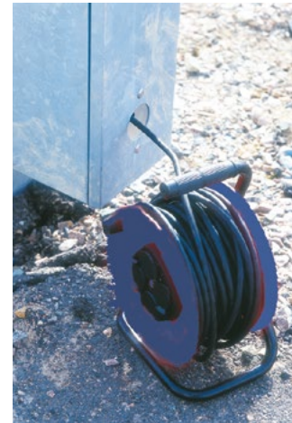
The openings on the sides of the cabinet is used for temporary power outlets, etc.
