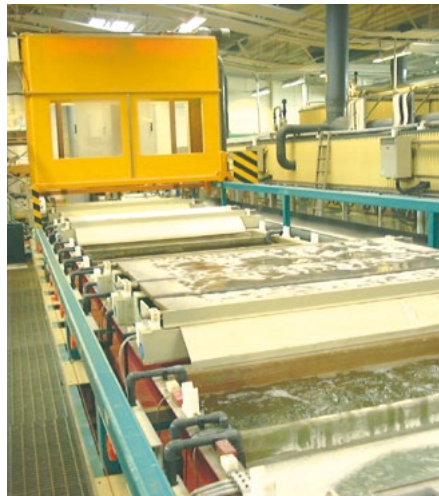
Automatic hot-dip galvanizing plant.
