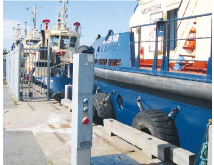
Distribution board at a port situated in Sweden.
