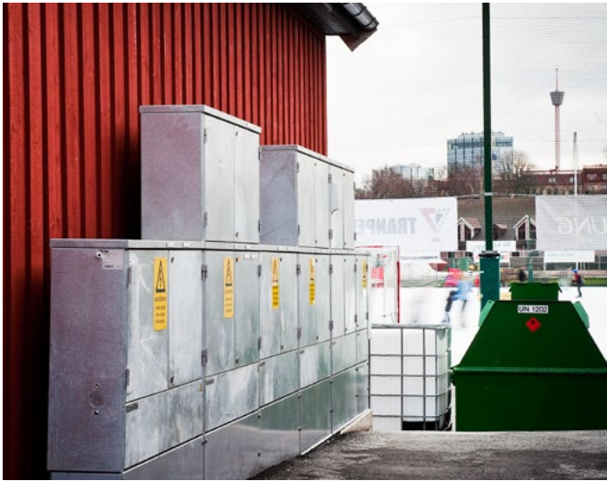
Cable distribution boards at Hedens bandy rink, Gothenburg, Sweden.
