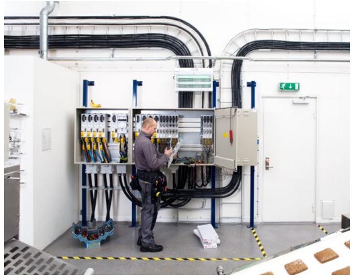
Distribution board in powder coated enclosure mounted on the wall in a switchgear room at a bakery, in Gothenburg, Sweden.
