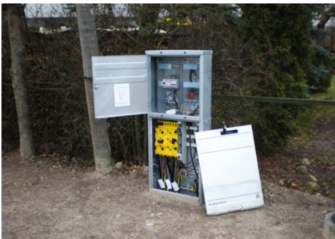
Enclosure with upper section CDCM used as metering cabinet, Latvia.
