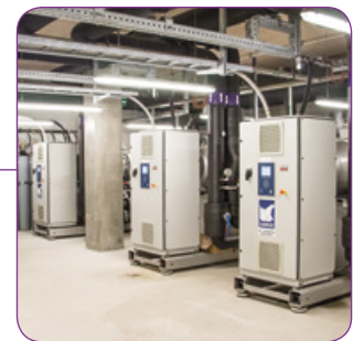
Complete chiller plant
