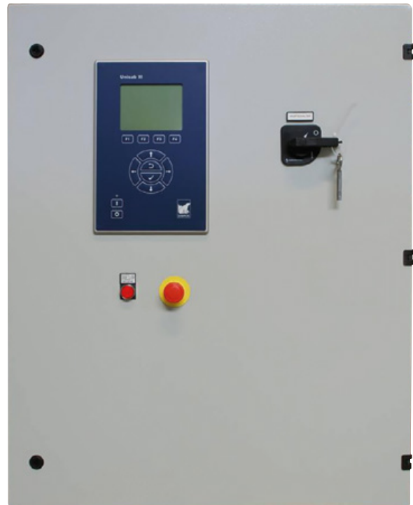
Sabroe Y/D starter panel
